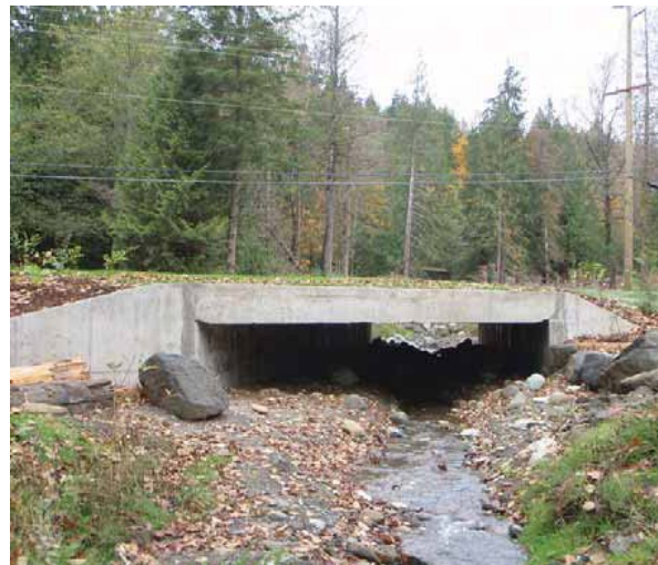
Source: WSDOT. A new box culvert replaced a small culvert on SR 542.
